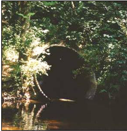
Photo 25: Cedar Creek Before - undersized and impaired Battleground Railroad culvert.
