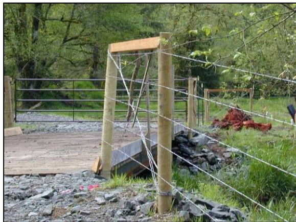
Photo 36: South Fork Chelatchie Creek After new bridge, expanded grazing area, and stream fencing.
