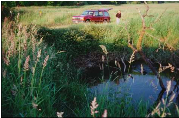
Photo 6: Lockwood Creek Before - existing culvert poorly functioning.
