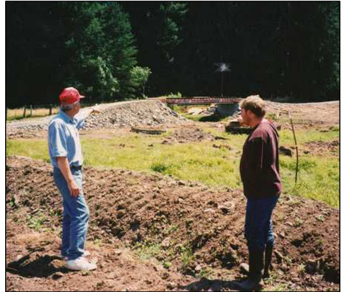
Photo 37: South Fork Chelatchie Creek during construction – cattle bridge, re-vegetation, and stream fencing.
