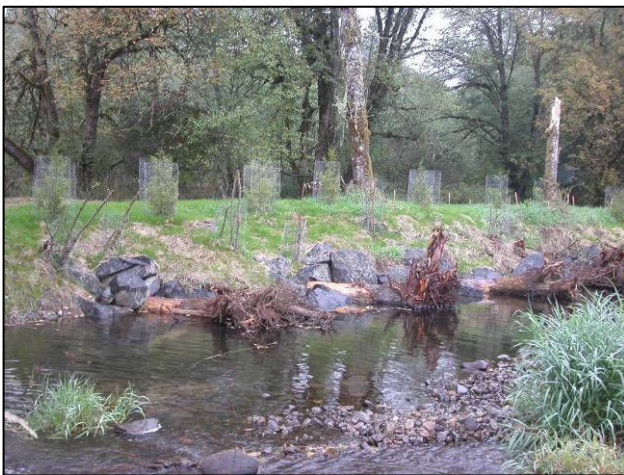
Photo 12: Cedar Creek After construction using root wads, cross veins, and re-created spawning beds and deep pools.
