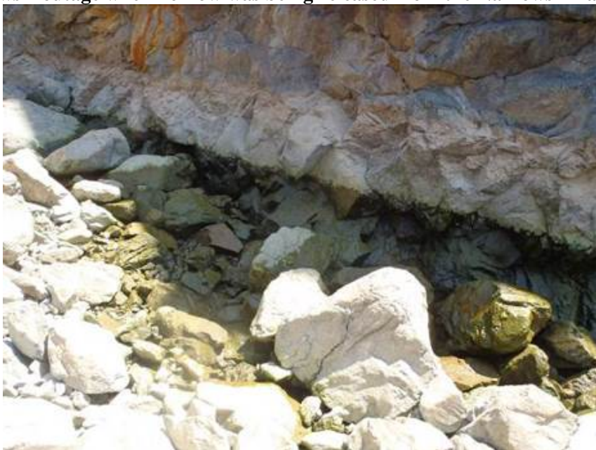
Figure 3.1-2. Picture of dry existing isolation pool depression on which the work would occur. The photo was taken during a Narrows 2 outage when no flow was being released from the Narrows 2 Facilities 33
