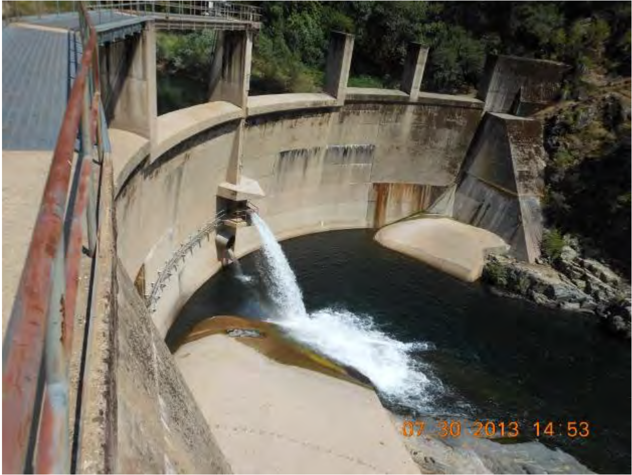
Figure 2.2-1. View to east of downstream face of Our House Diversion Dam. The majority of discharge shown in the photograph is through the fish release valve. A minor amount of gate leakage is occurring through the low level outlet valve, which is below the minimum flow release valve.
