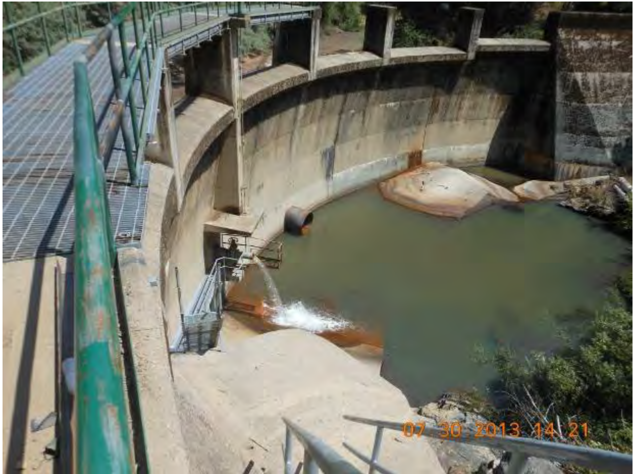
Figure 2.1-1. View to the east of the downstream face of Log Cabin Diversion Dam. The majority of discharge shown in the photograph is through the fish release valve. The low level outlet valve is to the right of the fish release valve.
