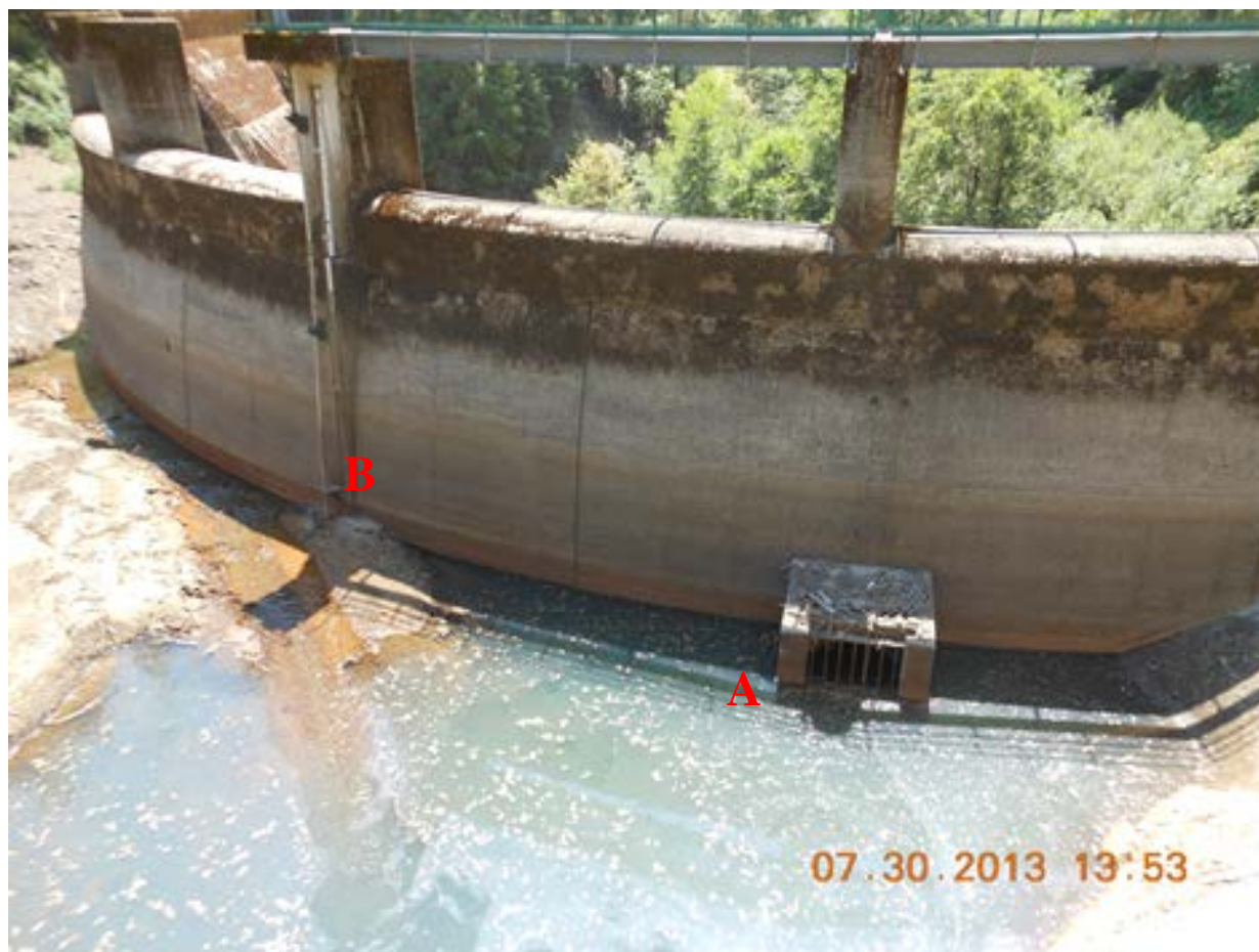
Figure 2.2-2. View to southwest of the upstream face of Log Cabin Diversion Dam. The intake for the fish release valve is marked by an “A;” the intake for the low level valve is marked with a “B.”
