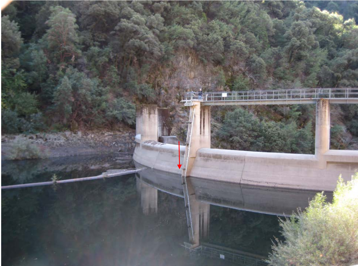
Figure 2.1-2. View to the south of upstream face of Our House Diversion Dam. The inlets for the low level valve and the fish release valve are located below the operator for the Low Level Valve, as indicated by the arrow in Figure 2.1-2.
