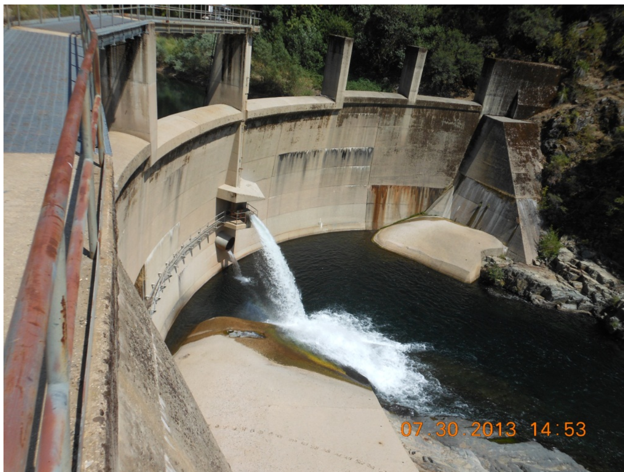
Figure 2.1-1. View to east of downstream face of Our House Diversion Dam. The majority of discharge is through the fish release valve. A minor amount of gate leakage is occurring through the low level outlet valve, which is below the minimum flow release valve.
