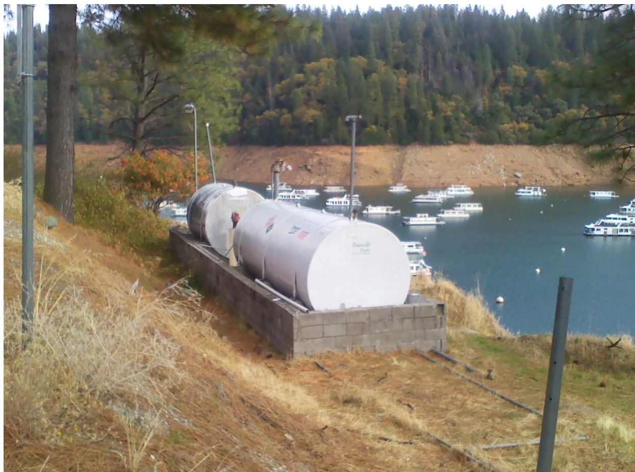
Figure 3.1-1. Photograph of Emerald Cove Marina fuel storage tanks.
