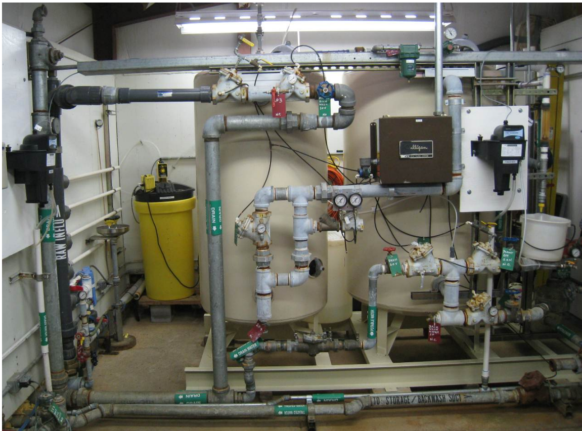
Figure 3.1-18. Representative photographs of the water treatment facility.
