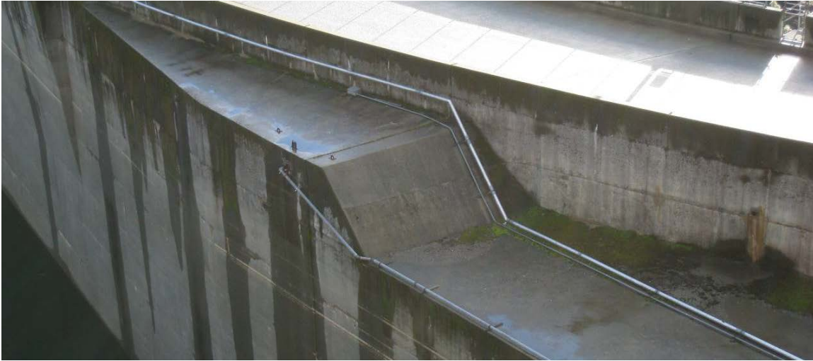
Figure 3.1-20. Representative photograph of the water distribution system across New Bullards Bar Dam.
