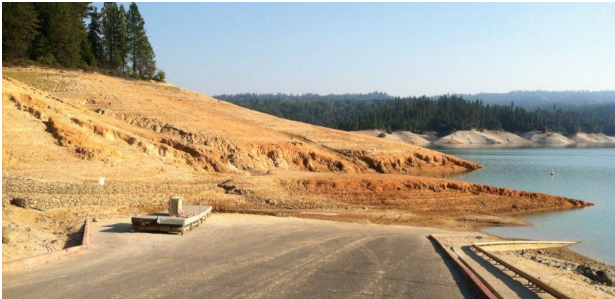
Figure 3.3.6-2. Photograph of the slope instability site upslope from the Dark Day boat ramp at low water levels (typically during the non-peak season). 21
