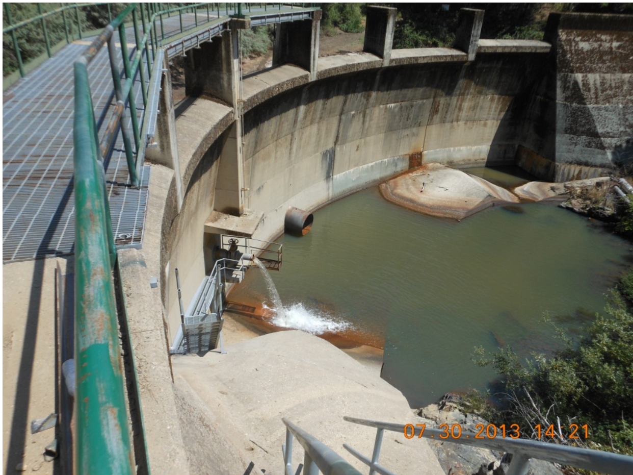
Figure 2.1-1. View to the east of the downstream face of Log Cabin Diversion Dam. The majority of discharge shown in photograph is through the fish release valve. The low level outlet valve is to the right of the fish release valve.
