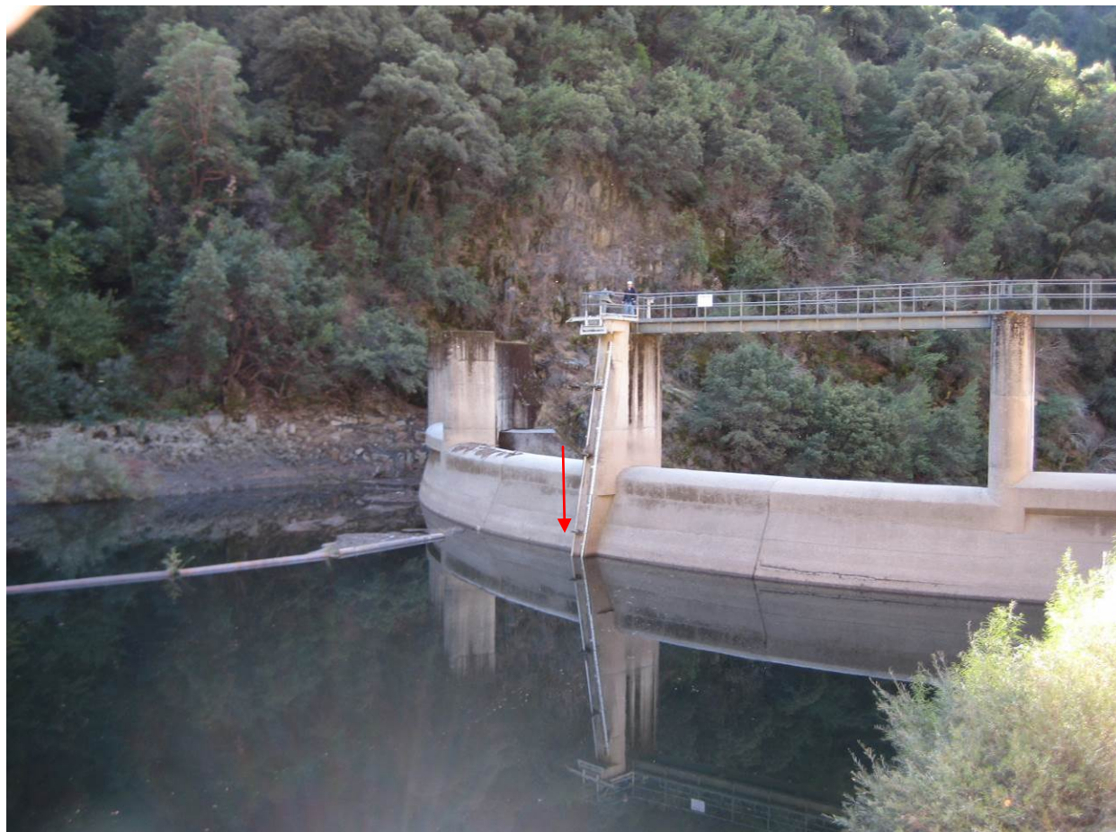
Figure 2.2-2. View to the south of upstream face of Our House Diversion Dam. The inlets for the low level valve and the fish release valve are located below the operator for the Low Level Valve, as indicated by the arrow above.
