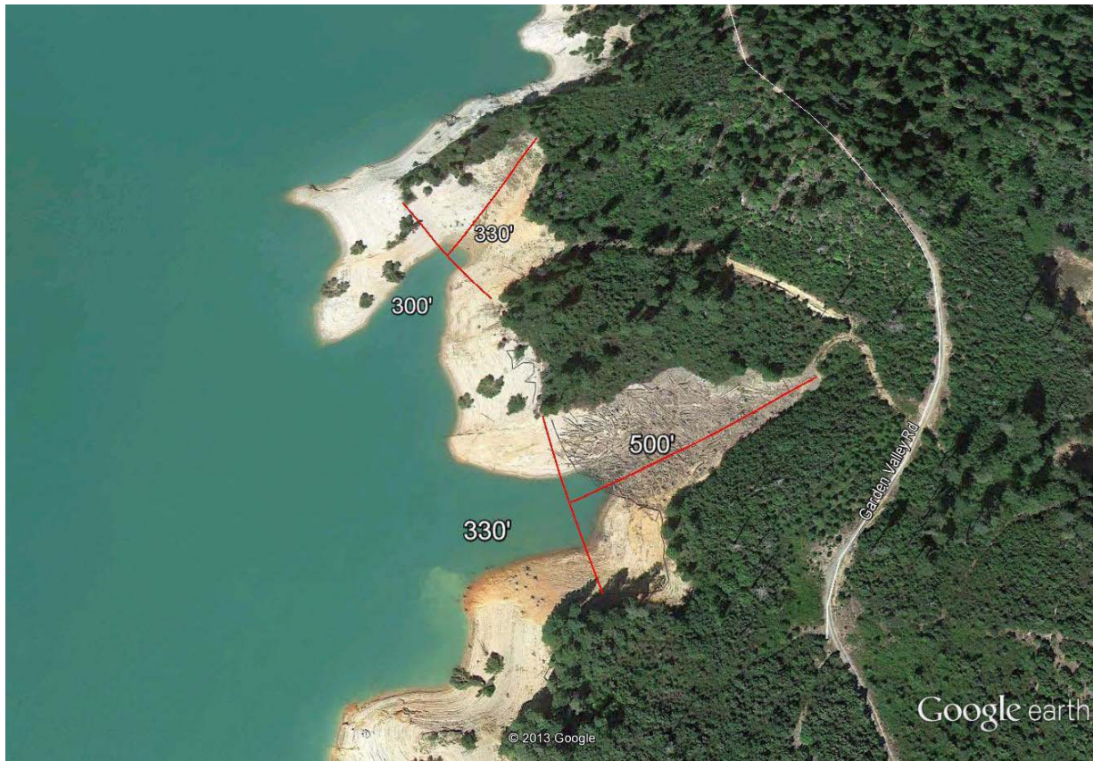
Figure 2.2-2. Coves 1 and 2 with the log booms in place and material stored in Cove 1.
