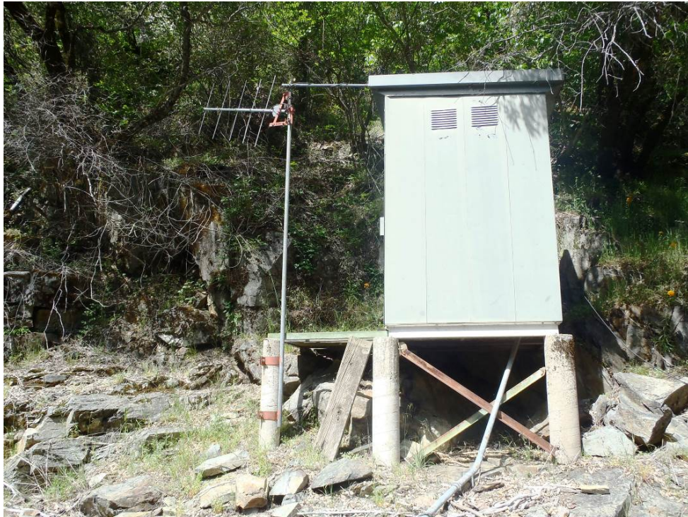
Figure 3.1-1. Middle Yuba downstream From Our House Diversion Dam gage shelter.
