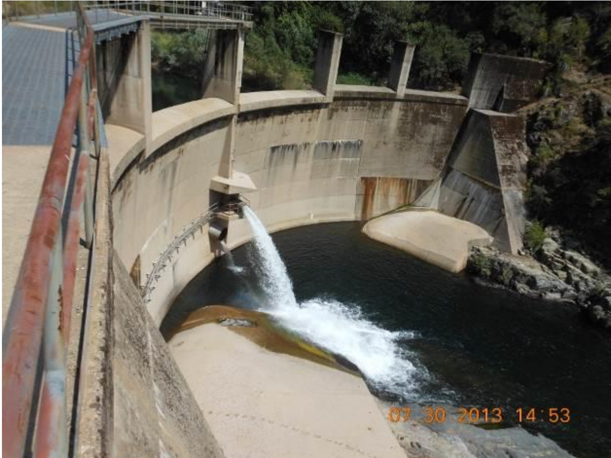
Figure 2.2-1. View to east of downstream face of Our House Diversion Dam. The majority of discharge shown in photograph is through the fish release valve. A minor amount of gate leakage is occurring through the low level outlet valve, which is below the minimum flow release valve.
