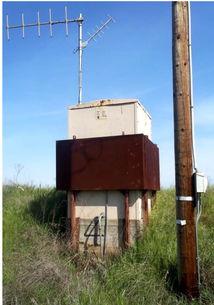
Figure 3.1-8. Yuba River downstream from Narrows 2 Powerhouse – Marysville gage shelter.
