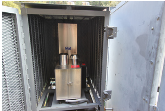
E) Propane powered (thermoelectric) generator runs the detection center from an onsite propane tank.
